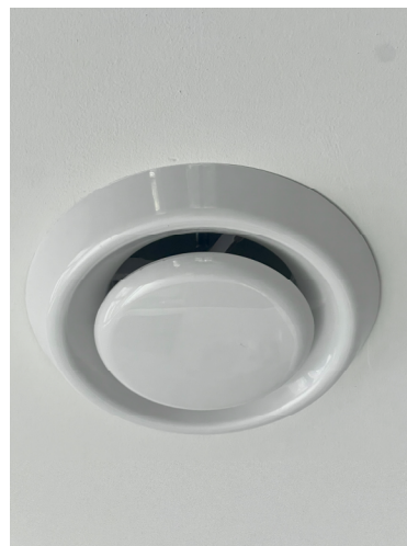
Kitchen and Bathroom Vent
