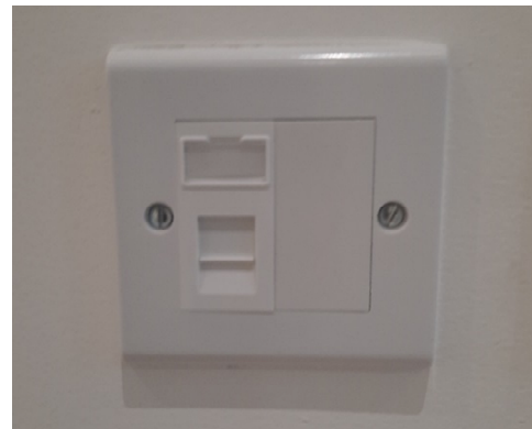
Telephone outlet in living area
