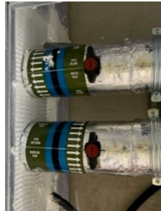
Image: Isolation valves
