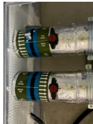
Image: Isolation valves
