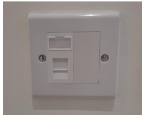
Telephone outlet in living area
