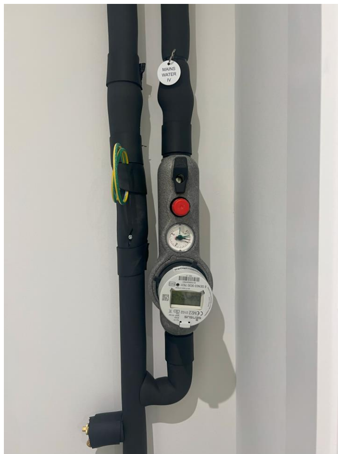
Water Meter and Valve
