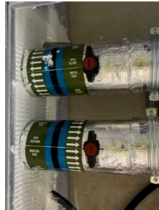
Image: Isolation valves
